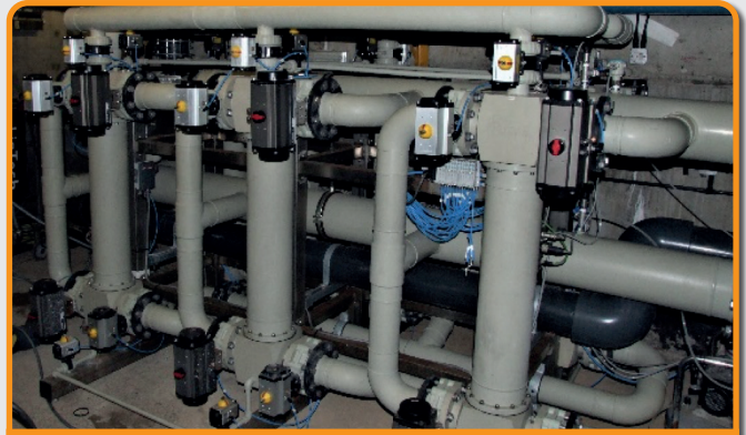
Six membrane system installed
