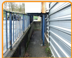
Restricted access to plantroom
