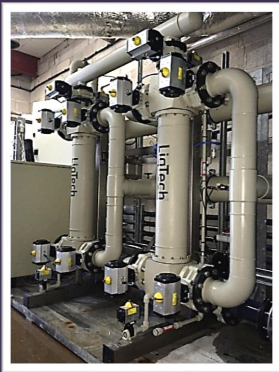
Figure 1 – The 2-membrane system at Alvaston Hall
